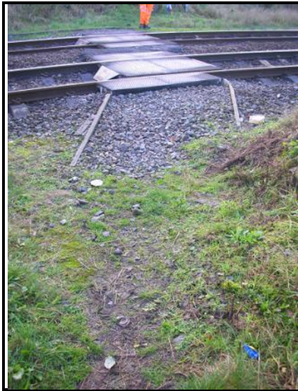
Figure 17: Ground condition approaching Moss Lane footpath crossing from the north. November 2013
