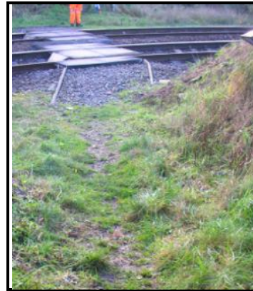
Figure 16: View of footpath surface approaching the crossing, after passing through the wicket gate. November 2013
